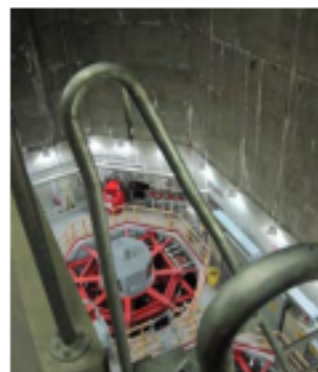
The Lake Hodges Pumped Storage Facility is part of the ESP and has the ability to generate energy.
