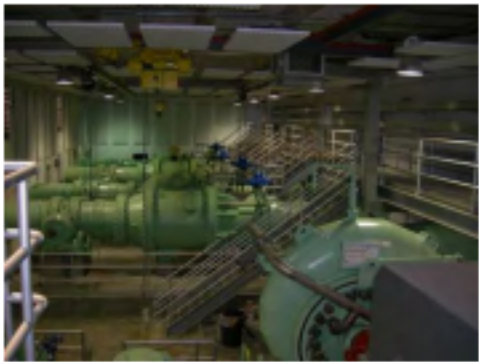
The Rancho Peñasquitos Pressure Control and Hydro Facility regulates flow to and from the San Vicente Reservoir.
