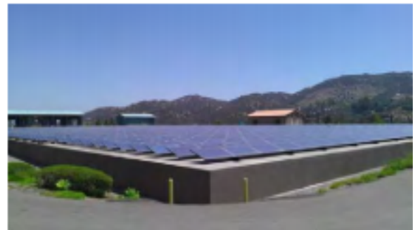
The Water Authority has identified various solar opportunities to supplement its renewable energy portfolio, similar to the solar panels installed at the Twin Oaks Valley WTP.
